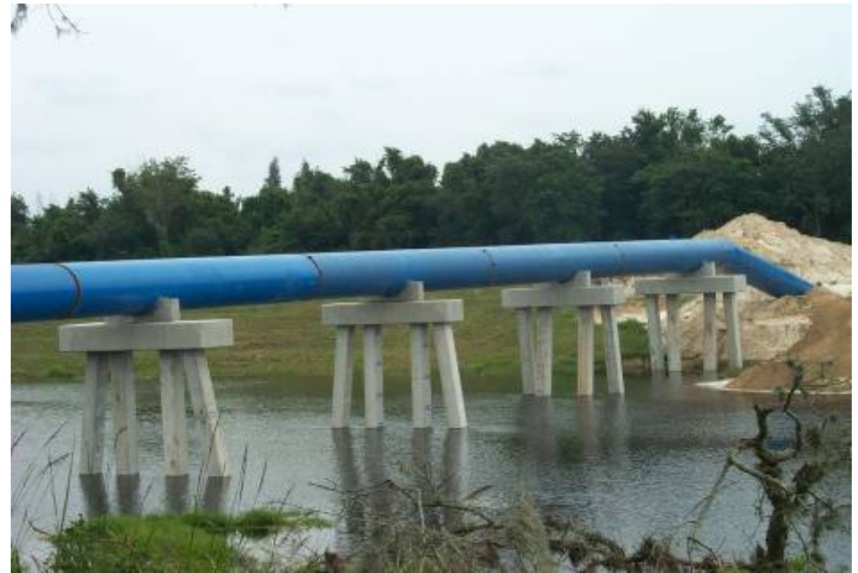
Large Diameter Pipelines
